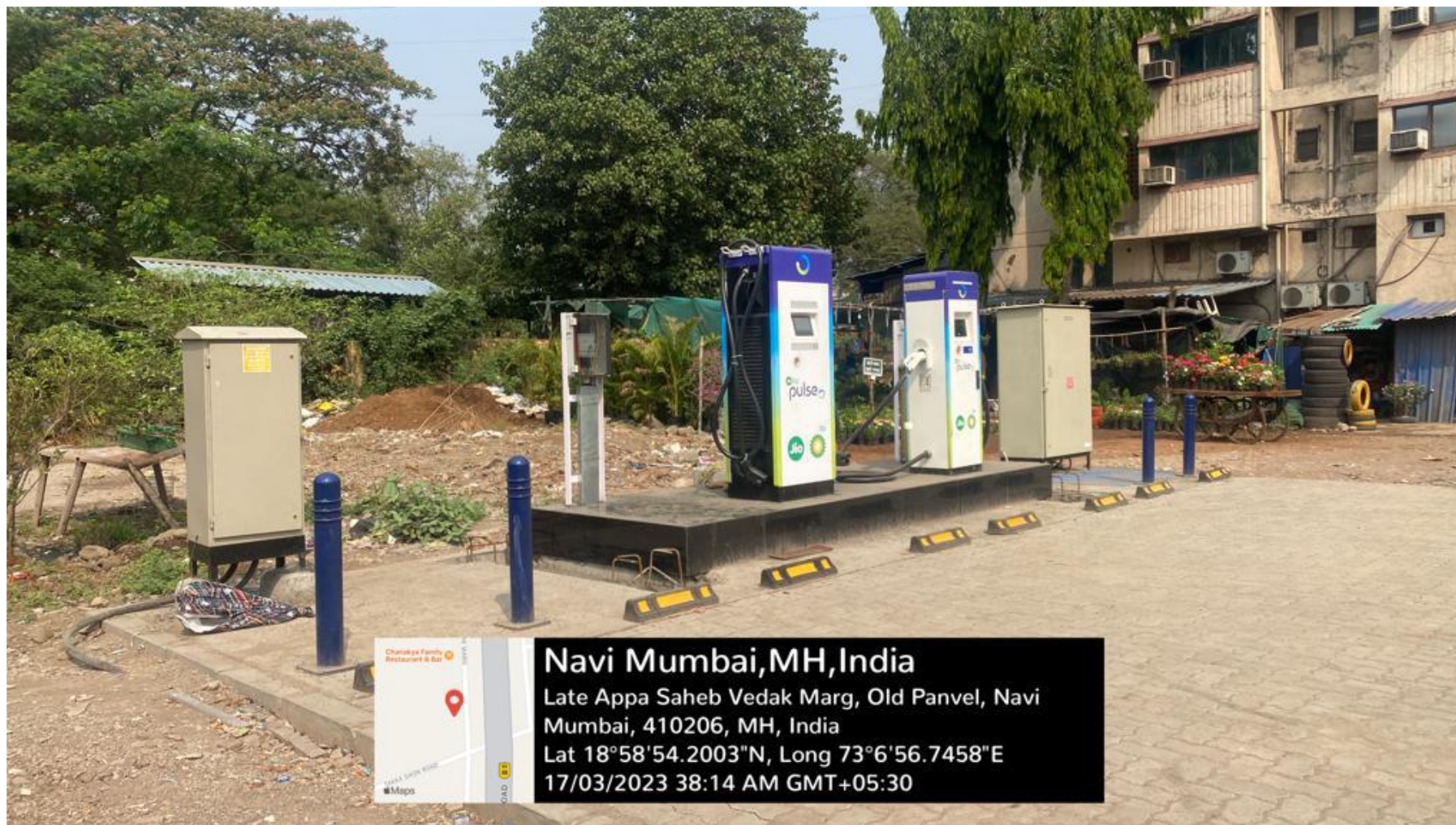
Panvel Municipal Corporation Installed EV Charging points
